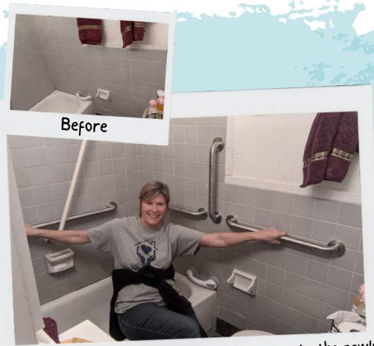
Good Neighbors Helping Hand. Lori Corner. puts the newly installed grab bars to the test. Safe and strong!
